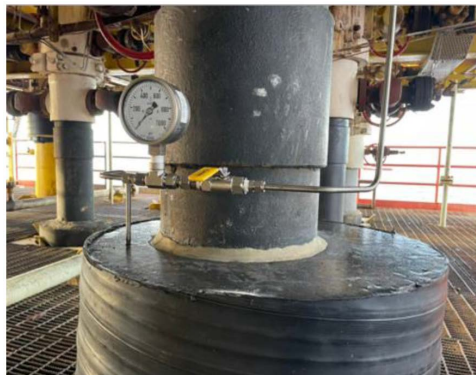
Figure 16(g)—Successful composite repair work using epoxy grout chemical sealant with tubing diverter installation for pressure management.
