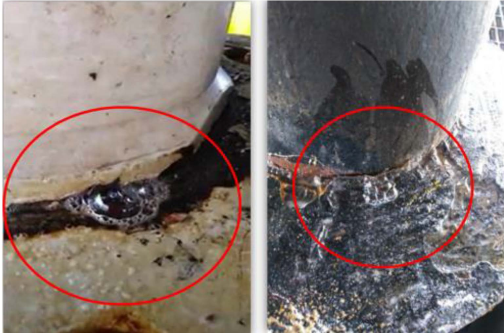
Figure 16(b)—Active gas emission at conductor surface area for well C1 and C2.
