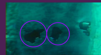
Underwater images of actual repairable leaks of various sizes
