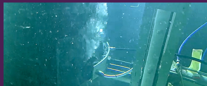
Once the metal sealant has cured, piston is released. Metal plate remains in place ready for the Helicoid Epoxy Sleeve ® to be installed.
